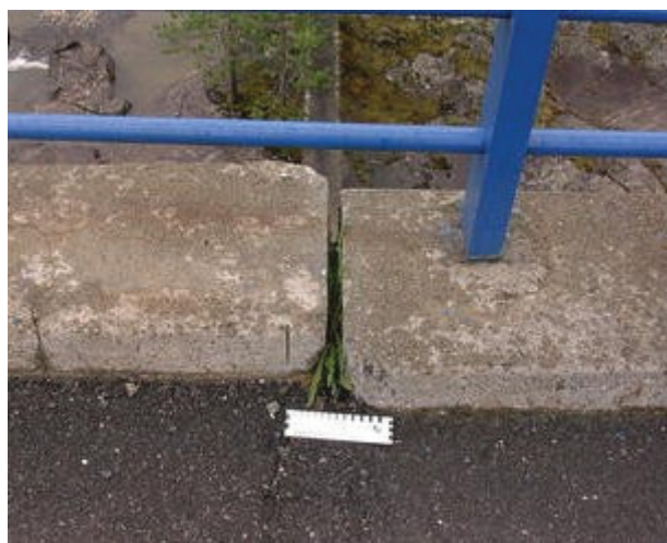
Figure 2.8. Misalignment in the crest of a concrete dam due to ASR (Fernandes and Broekmans 2013).
