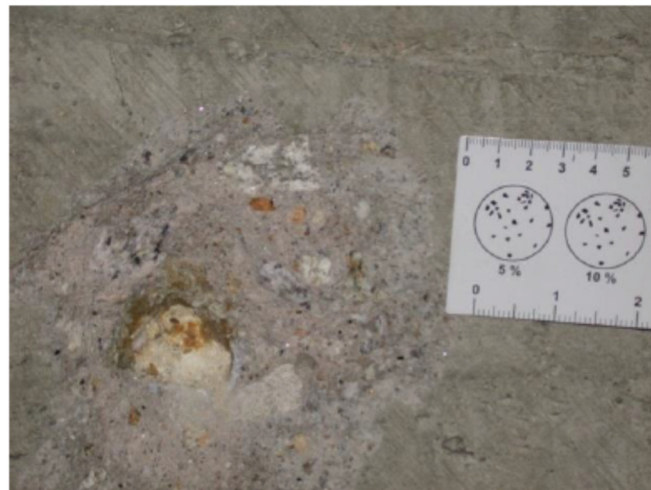
Figure 2.10. Example of pop-out in a concrete element (Ramos, 2013).
