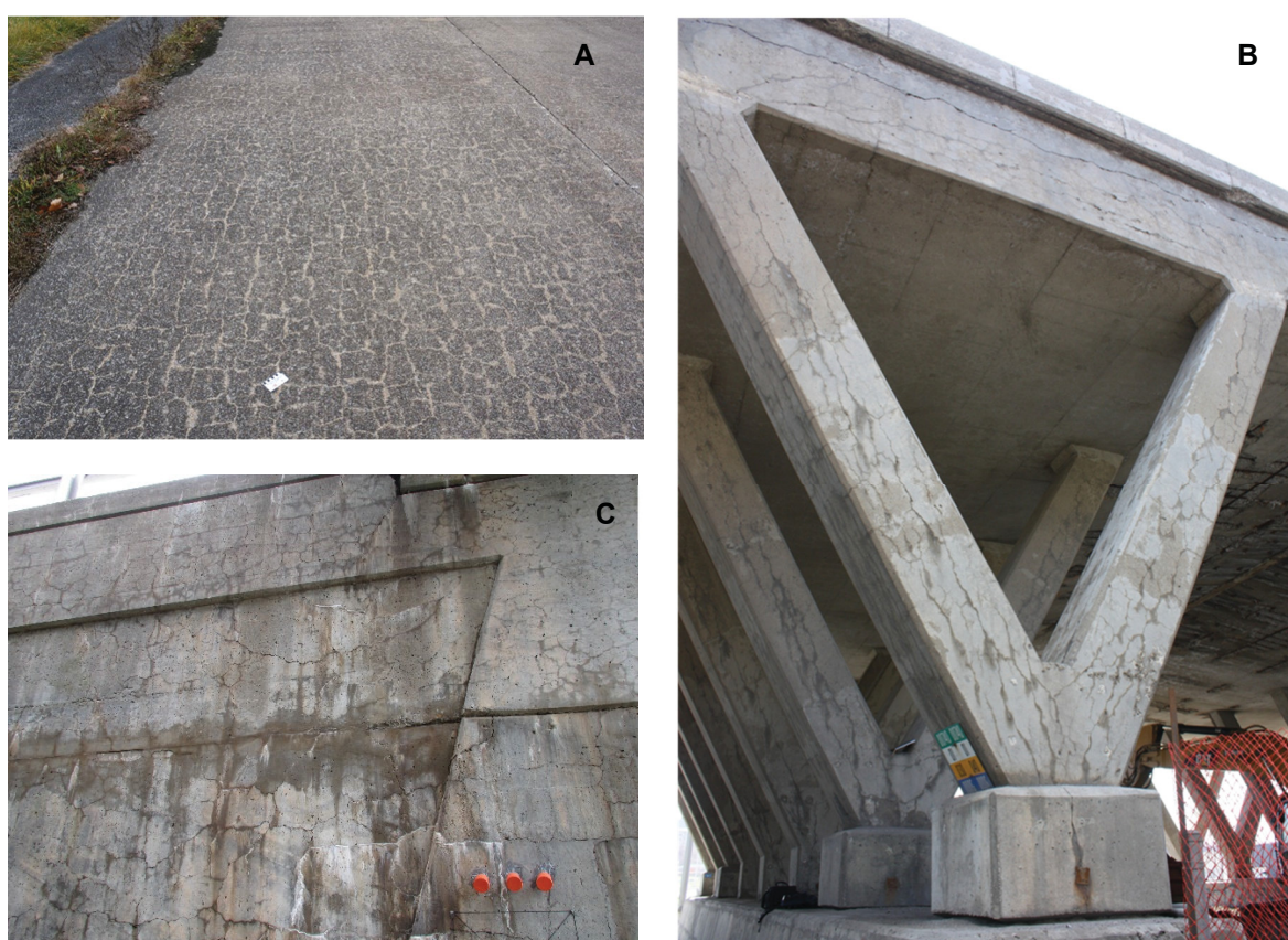
Figure 2.7. Patterns of cracking in concrete due to ASR: (A) map-cracking in concrete pavement, (B) Map cracking in the wing wall of a highway bridge structure, and (C) longitudinal cracking following the main reinforcement in columns of a highway concrete structure (with compliments of B. Fournier).
