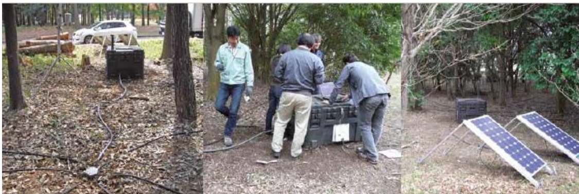
Photo 1.5 - Installation of CTBTO portable array in Tsukuba, Japan, in March 2010 (in Mialle et al. , 2010).
