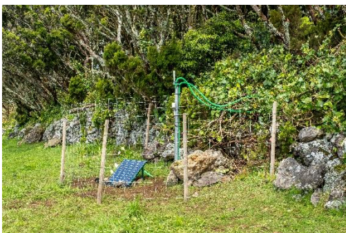
Photo B.33 - Fence protecting solar panel and communications mast from the cattle.
