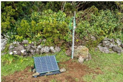
Photo B.25 - Solar panel and mast with GPS and GSM antennas.
