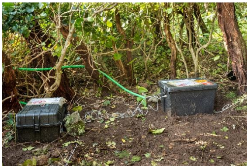
Photo B.47 - Communications (left) and energy equipment (right).
