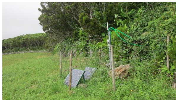
Photo B.34 - Optimizing the recharge of batteries with a second solar panel.
