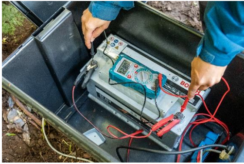
Photo B.35 - Energy box with 1 battery.
