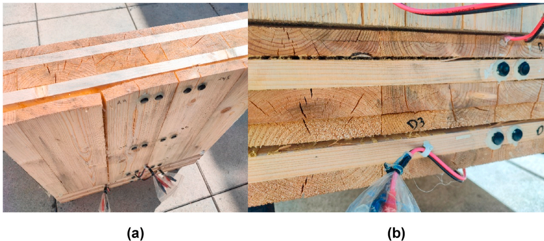
Fig. 8. Delamination, drying cracks, and deformations caused by repeated wetting and drying of the end-grain face: (a) Zone A; (b) Zone B. (colour). (For interpretation of the references to colour in this figure legend, the reader is referred to the Web version of this article.)
